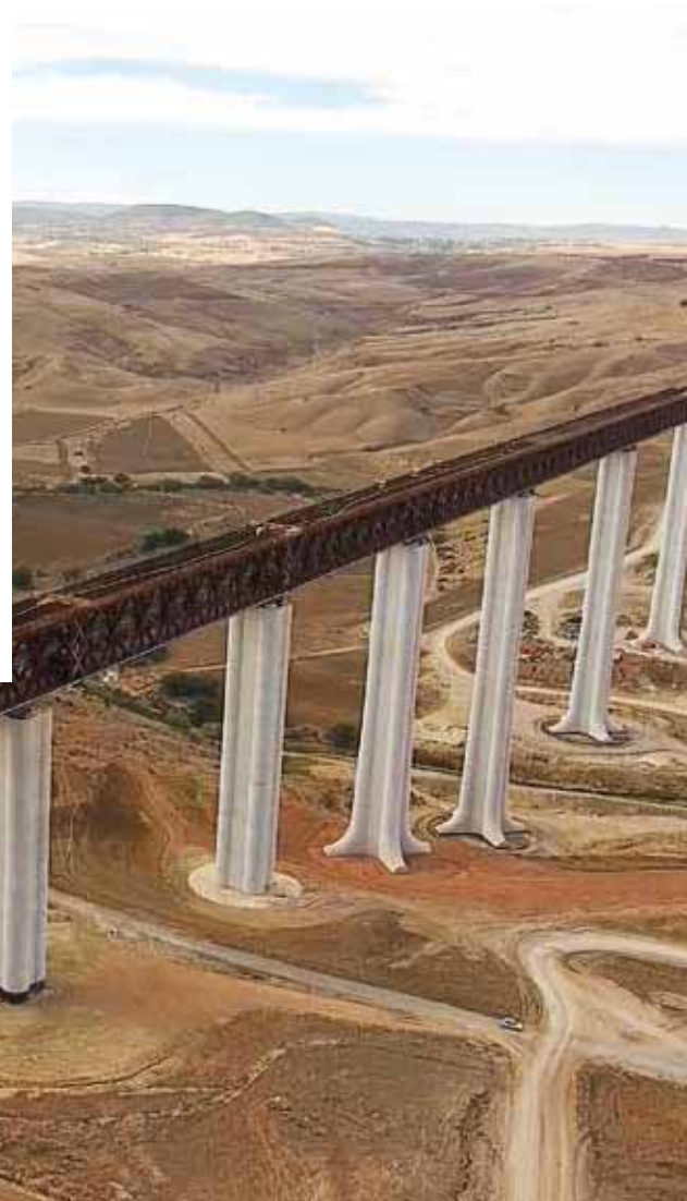
The great viaduct of Tlemcen Considered the greatest railway viaduct in Africa, Measuring 1780 metres in length
